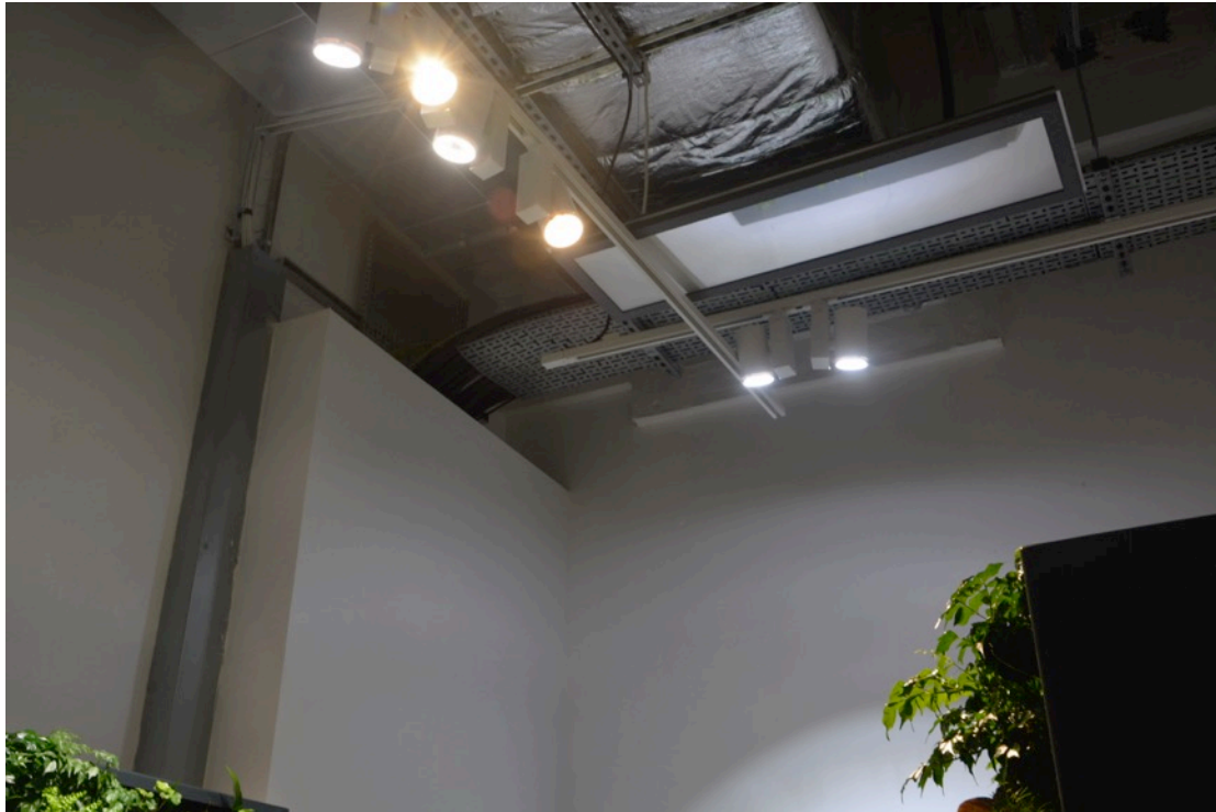
Figure 4: Luminaire arrangement in the ceiling for lighting the three green walls
